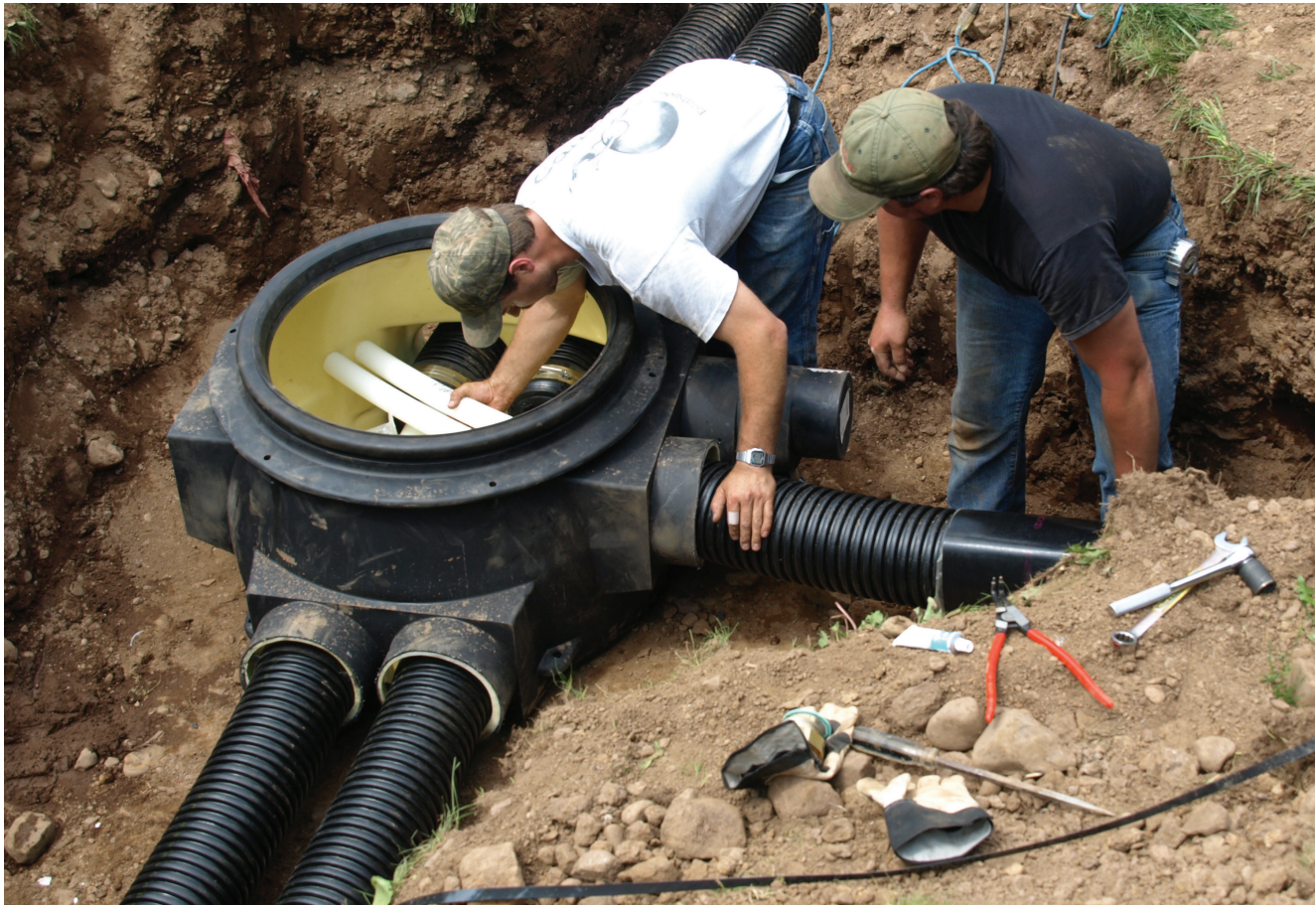
Figure 5-8: Ecoflex connection vault
