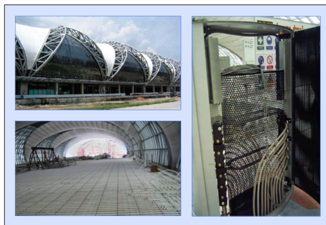
Figure 5: Installation of floor cooling with manifolds in the displacement diffusers at the new Bangkok airport.
